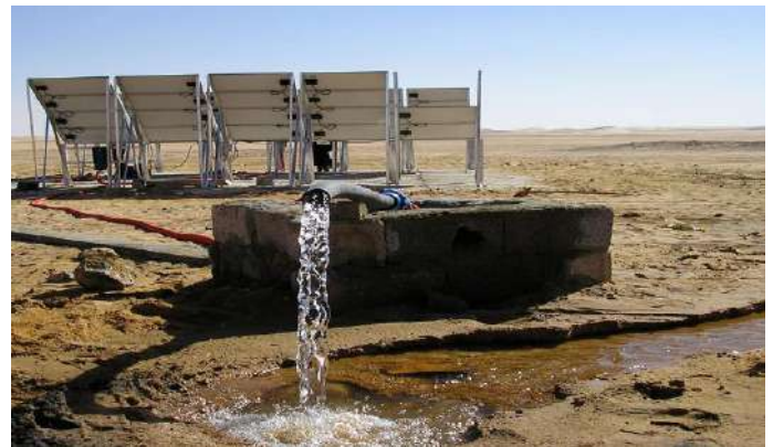
Fig. 7. PV Water Pumping Beer Tssawa
